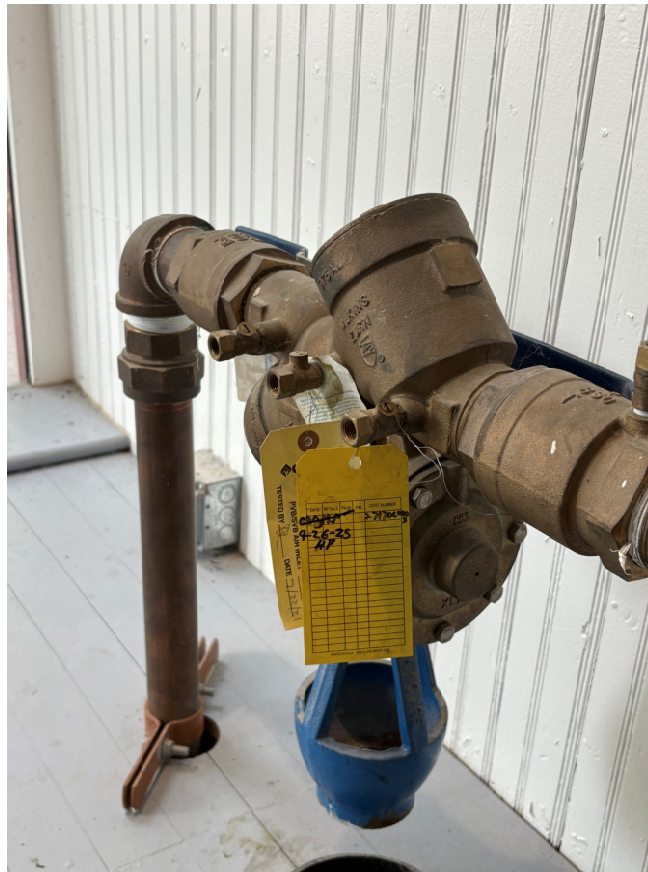
Photo-20 Interior 5 side floor 1 RPZ backflow preventer.
