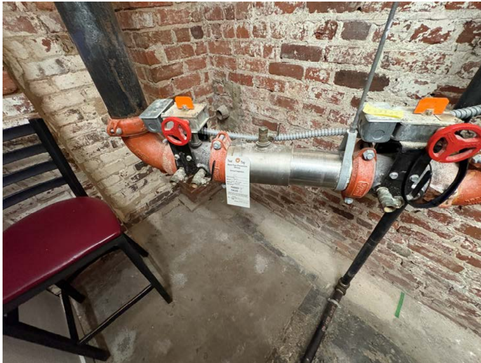
Photo-18 Interior basement fire sprinkler controls
